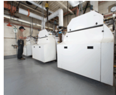
Clearfire boilers installed at the Denver Federal Center.
