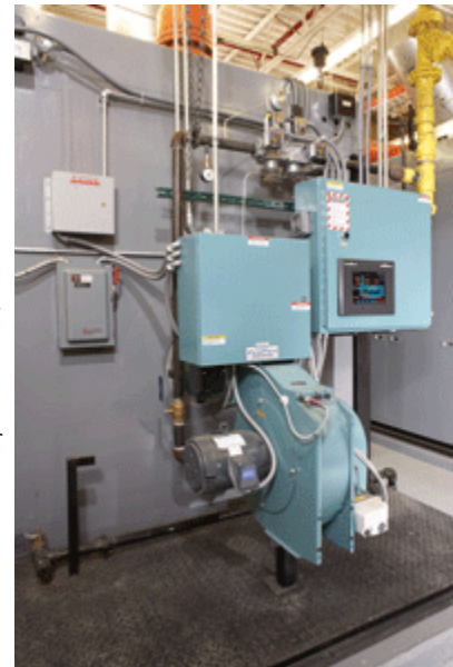
A retrofitted burner at the Denver Federal Center.
